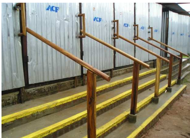
Modified latrines with standardized steps, handrails, a non-slippery surface, and yellow edges for visually-impaired people.
